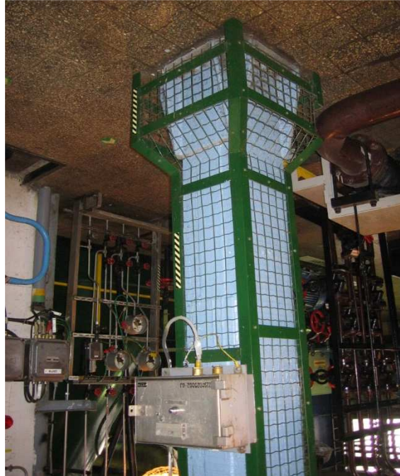
Figure 2.1.4-1: Additional passive fire protection of turbine oil tank support column
