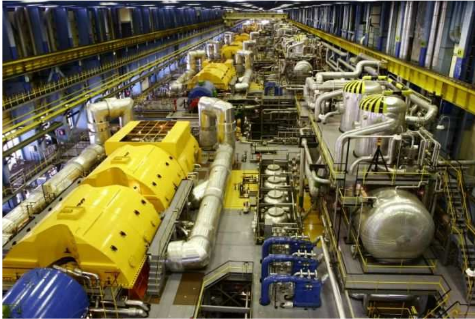
Figure 2.1.2 – 1: Turbine hall of the PAE
